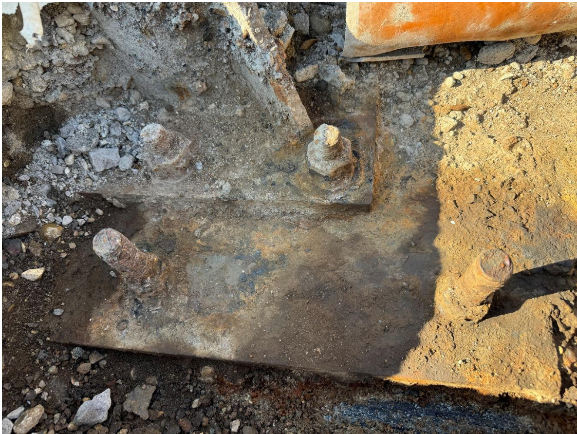
Figure 4- Corroded base for lamp column in Span 4- bolt not extracted
