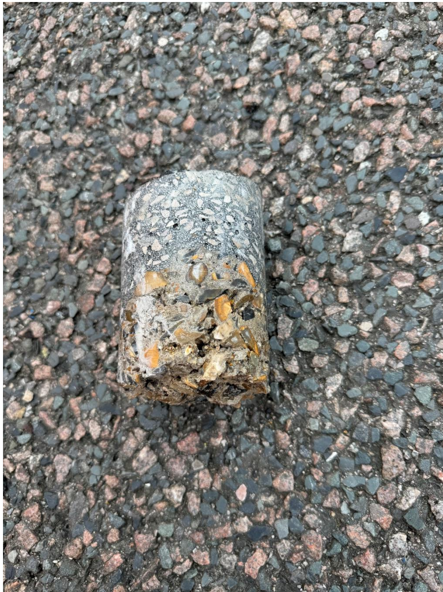
Figure 3- Core from deck topside showing poorly compacted parent concrete below repair.
