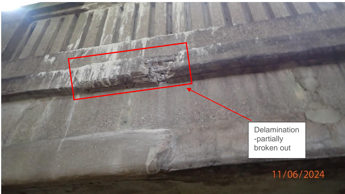
Figure 5 -Defect on parapet at northwest end
